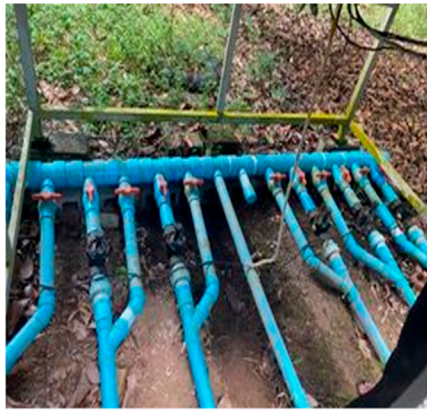
Automatic watering system
