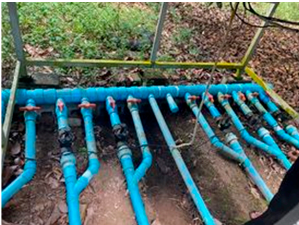
Figure 5: The 6-valves in the automatic water management system inside the mangosteen garden.
